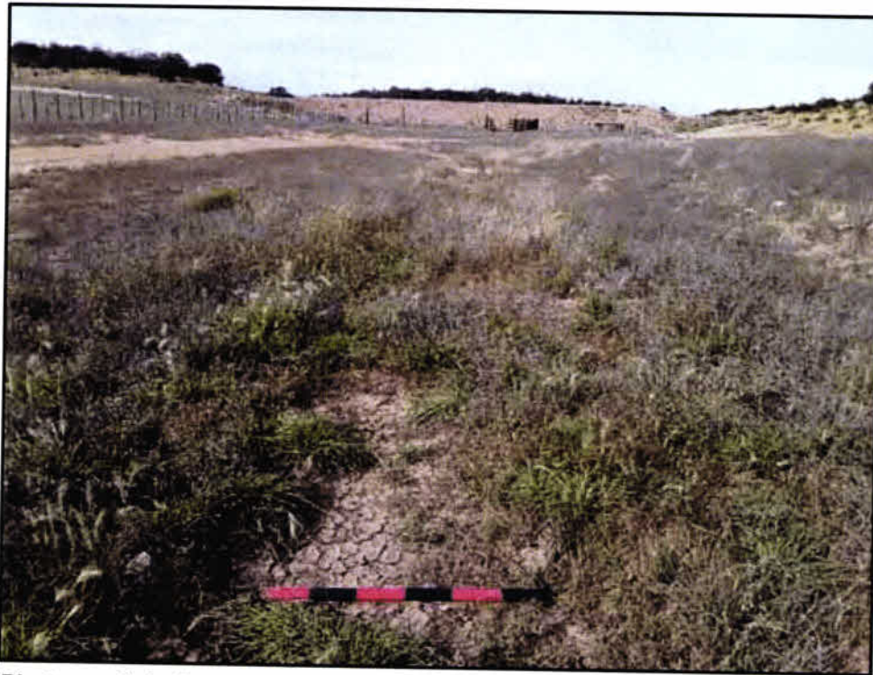
Photograph A.131. Lockwood Canyon (Feature 44), DP-67; swale/erosional feature influenced by livestock activity, view upgradient.
