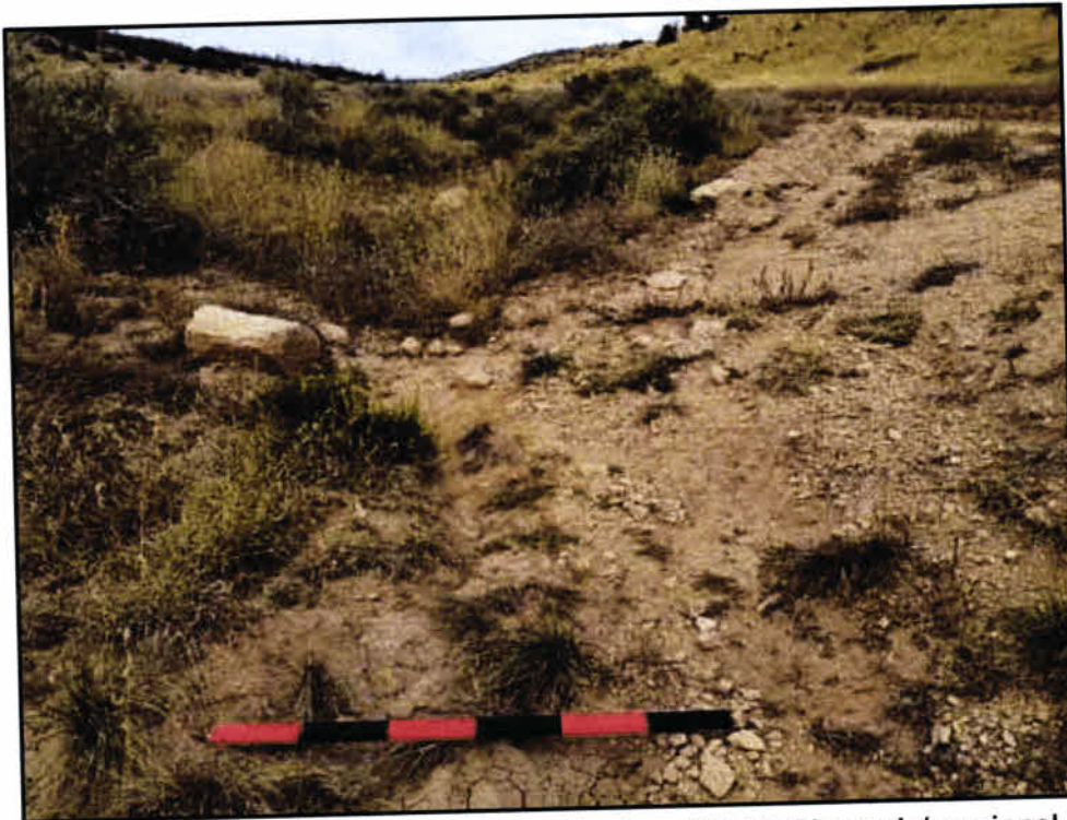
Photograph A.125. Lockwood Canyon (Feature 44), DP-63; swale/erosional feature influenced by livestock activity, view upgradient.
