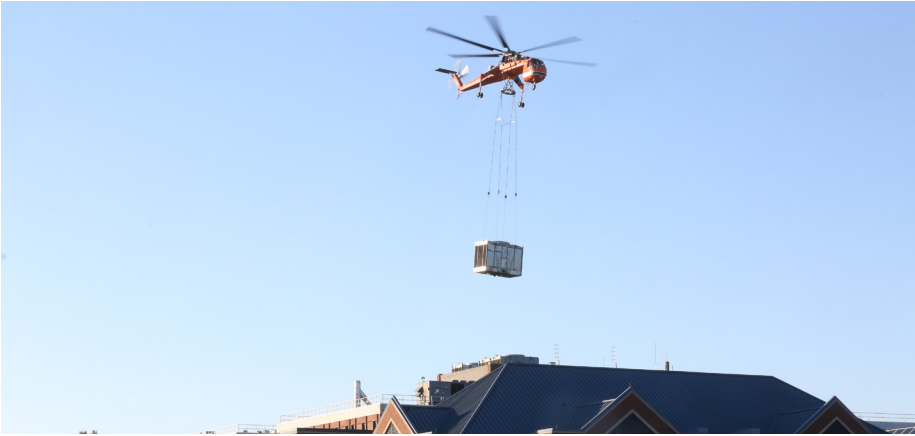
An air-crane was used to remove the older, failed cooling tower equipment off of the main hospital, building 200, and to install the new, energy efficient cooling tower equipment onto the roof.
