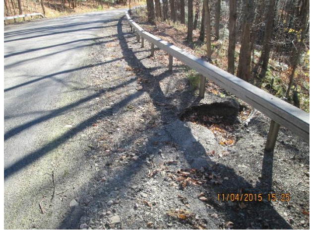
DETERIORATED AND WASHED OUT WEST SHOULDER
